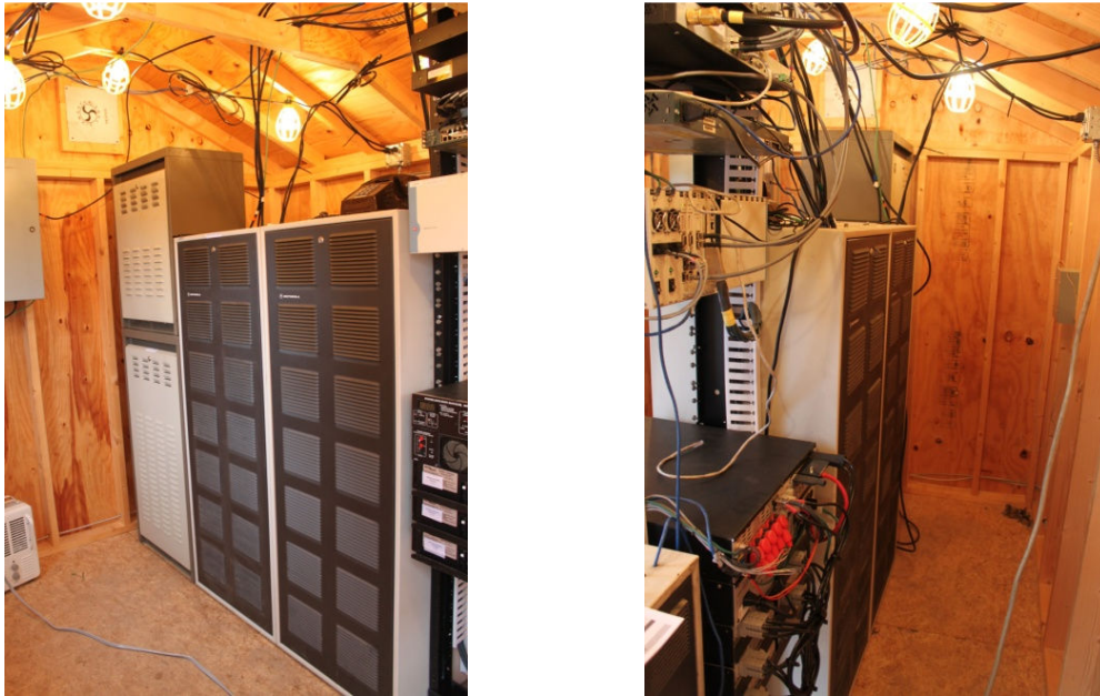
Figure 5-29: Airport Shelter (Site Abandoned)
