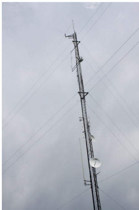
Figure 5-6: Hawkins Hill Tower
